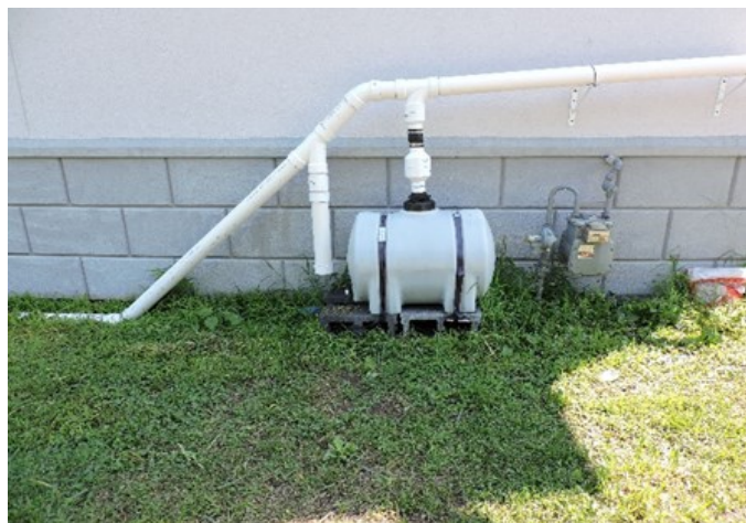
Photo C. First flush diversion tank.
