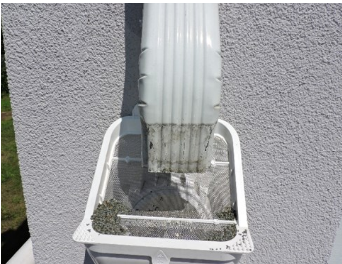
Photo B. Mesh filter on the rainwater collection system.
