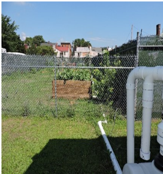
Photo D. Pipe connecting the rainwater collection and first flush components to the raised beds. The rainwater travels through the pipes due to the gravity of the slight downward slope.
