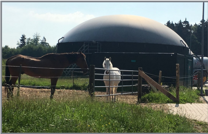
Upright anaerobic digester at a dairy farm in Stuttgart, Germany. Photo: Stephanie Lansing
