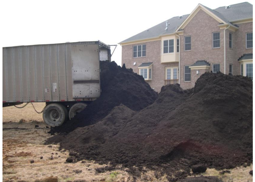
A walking floor tractor trailer, which holds 35 to 40 cubic yards, is often used to deliver compost to large job sites.
