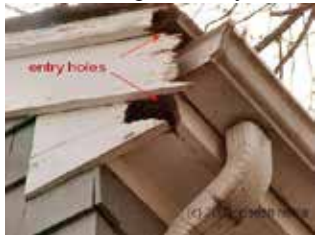
Squirrel damage on house
