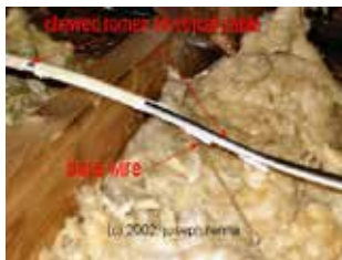
Squirrel damage in attic
