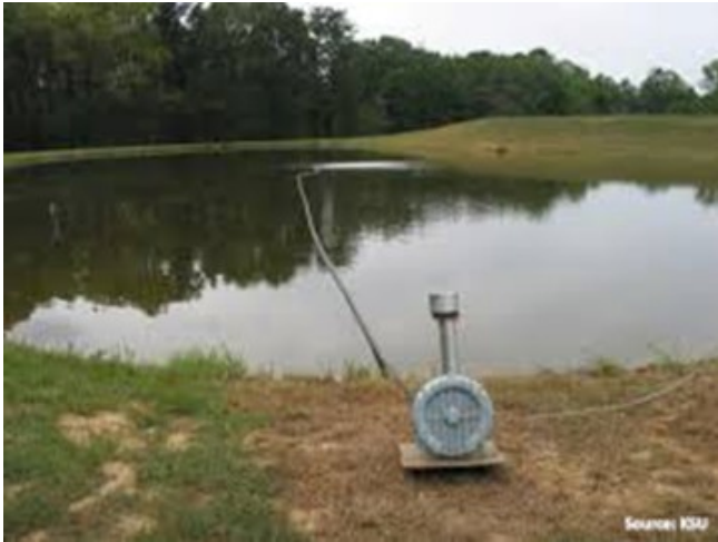
Figure 2. Diffused aeration in pond supplied by a regenerative blower.
