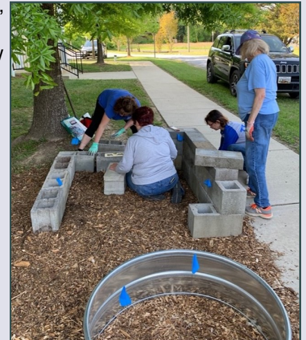
The fire ring is placed into position and a cinder block raised bed is built
