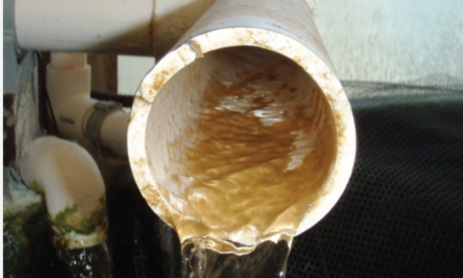
Figure 1: Pipe with a moderate biofilm.
