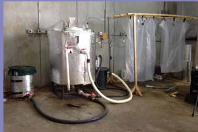
Top photo: Anaerobic digester
